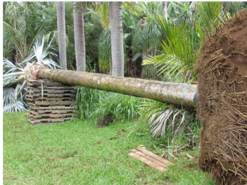
After the plywood box is carefully removed, a steel cable is drawn across the bottom of the root mass to form a flat bottom that allows for upright orientation in a quarantine nursery near the site of installation. Note fine roots at the side surface of the root ball.
